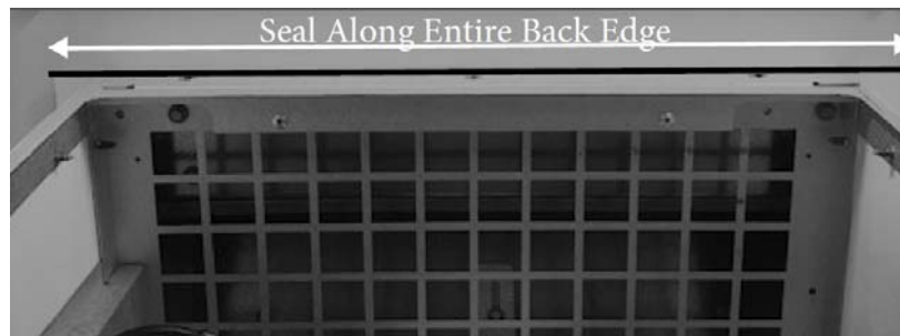
Seal Along back of Pressurization Module at Bard Unit
