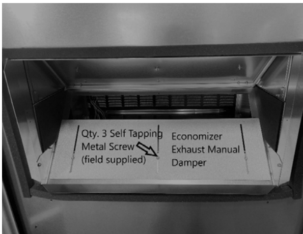
Economizer Exhaust Manual Damper (Bard Economizer Damper Adjusted Open)
