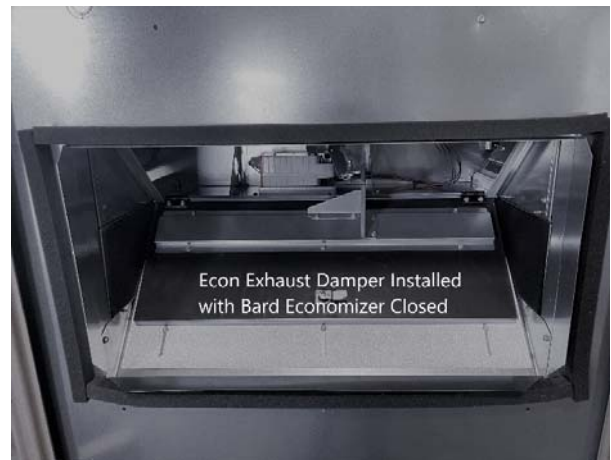
Bard Economizer Damper in Fully Closed Position
