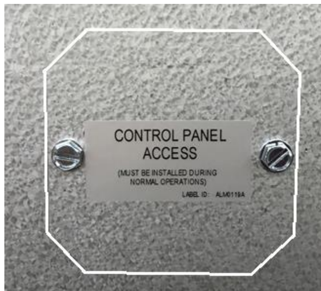
Figure 1 – Control Board Access
